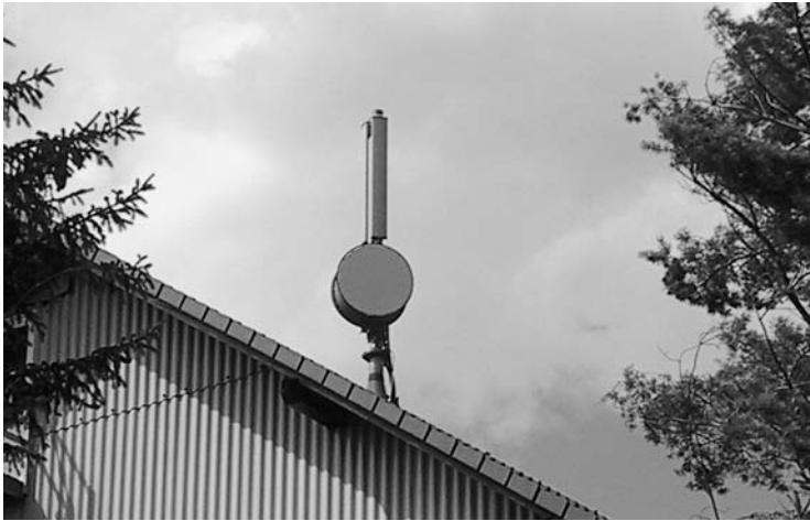
Figure 1.18 A typical antenna of a GSM base station. The optional microwave directional antenna (round antenna at the bottom of the mast) connects the base station with the GSM network
