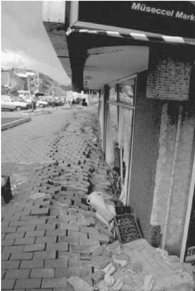
FIGURE 8.5 The building suffered a liquefaction-induced punching shear failure during the Izmit earthquake in Turkey on August 17, 1999. (Photograph from the Izmit Collection, EERC, University of California, Berkeley.)
