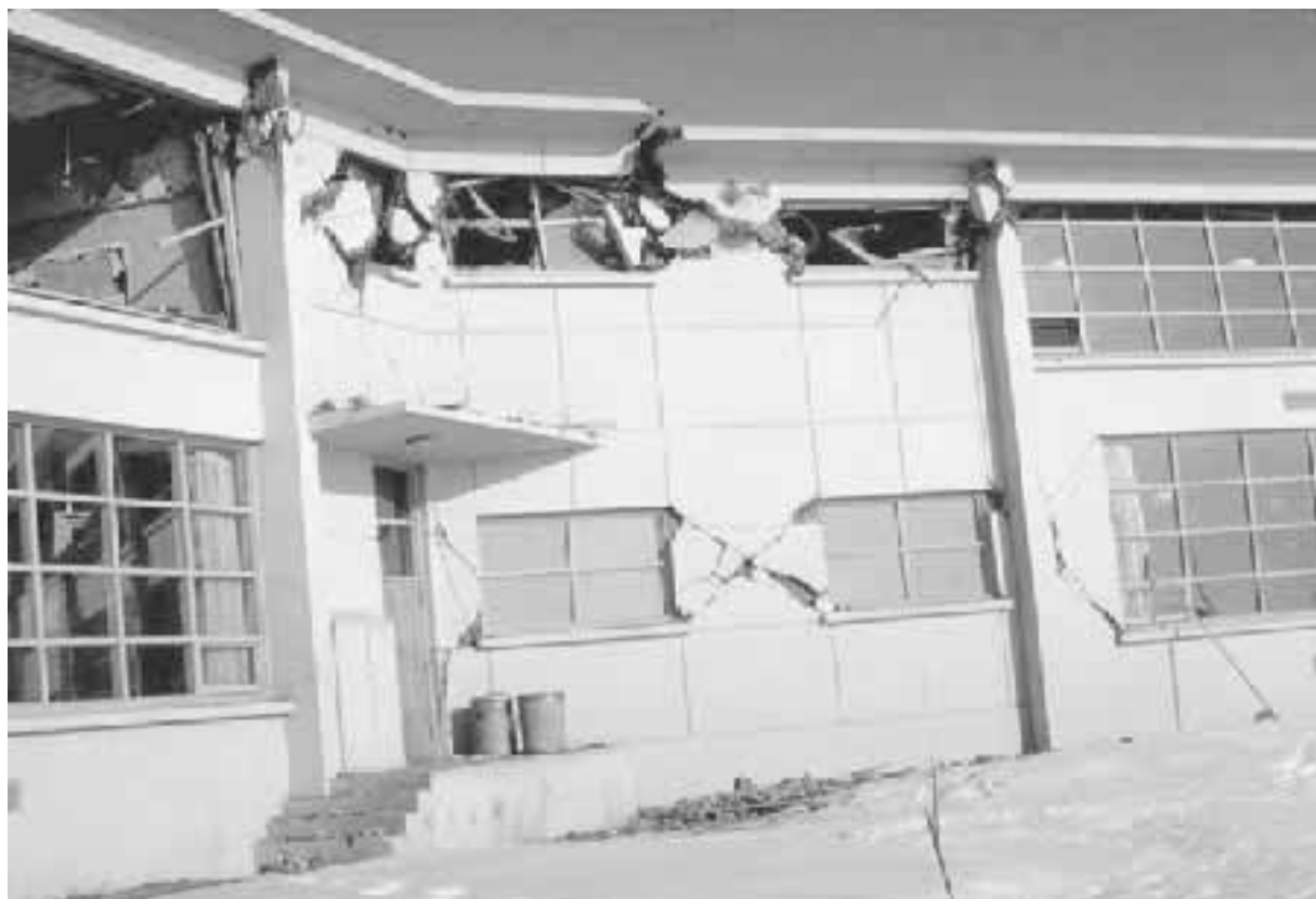
FIGURE 4.18 Damage to a shear wall at the West Anchorage High School caused by the Prince William Sound earthquake in Alaska on March 27, 1964. (Photograph from the Steinbrugge Collection, EERC, University of California, Berkeley.)
