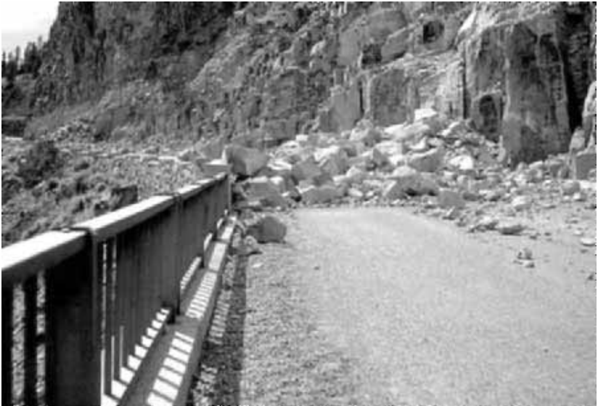
FIGURE 9.3 A large rockfall caused by the Hebgen Lake earthquake in Montana on August 17, 1959. (Photograph from the Steinbrugge Collection, EERC, University of California, Berkeley.)
