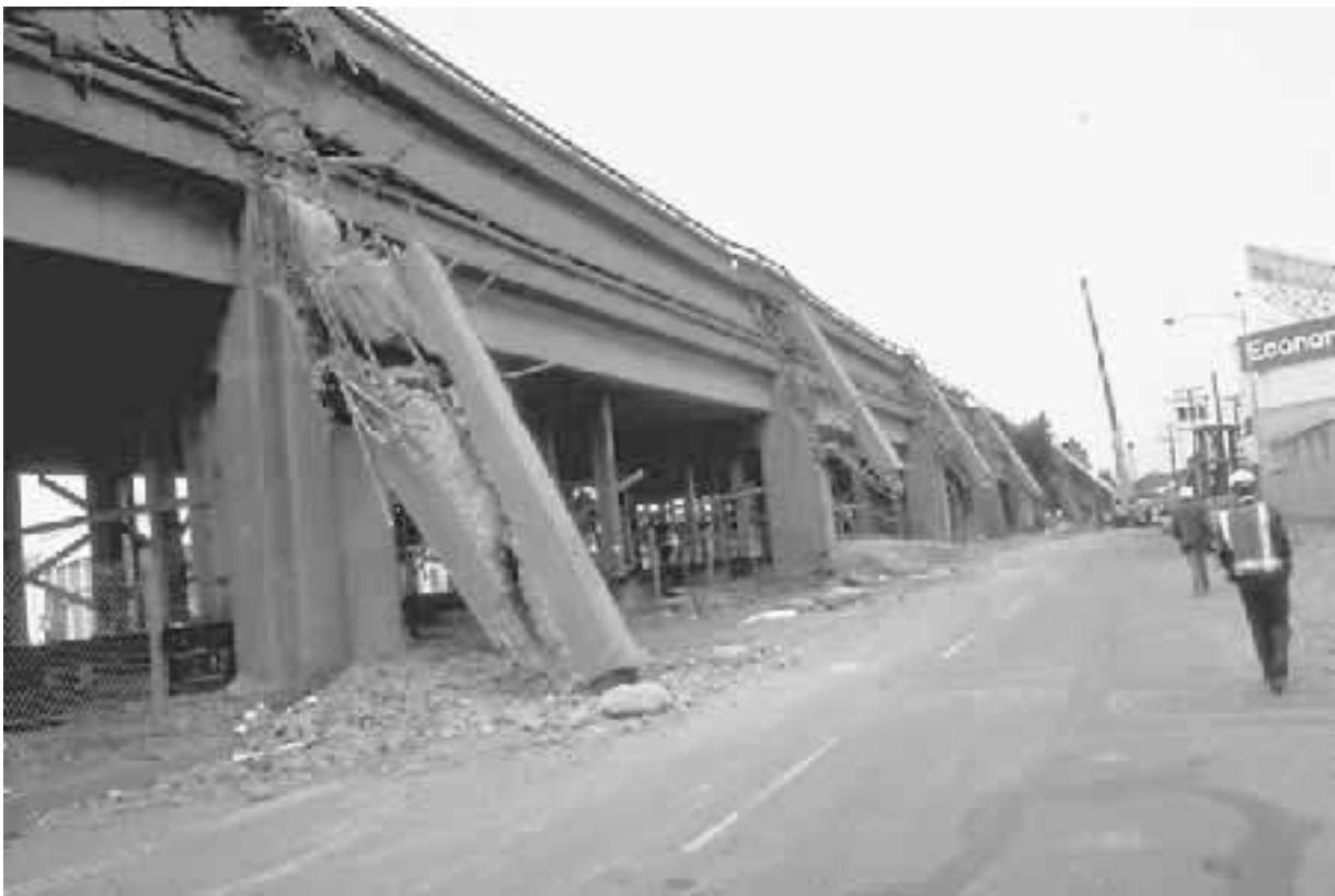
FIGURE 4.28 Close-up view of the collapse of the Cypress Street Viaduct caused by the Loma Prieta earthquake in California on October 17, 1989. (From USGS.)
