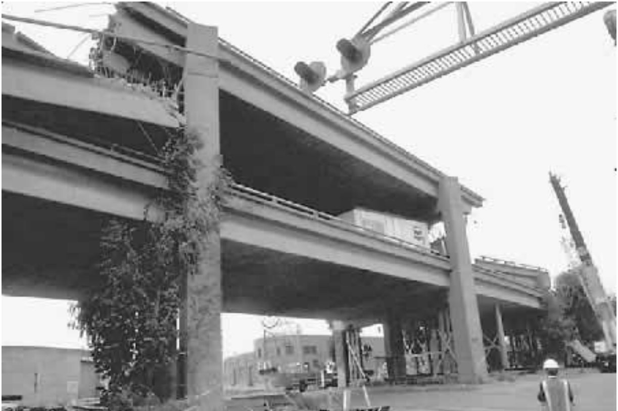
FIGURE 4.29 Close-up view of the collapse of the Cypress Street Viaduct caused by the Loma Prieta earthquake in California on October 17, 1989. (From USGS.)
