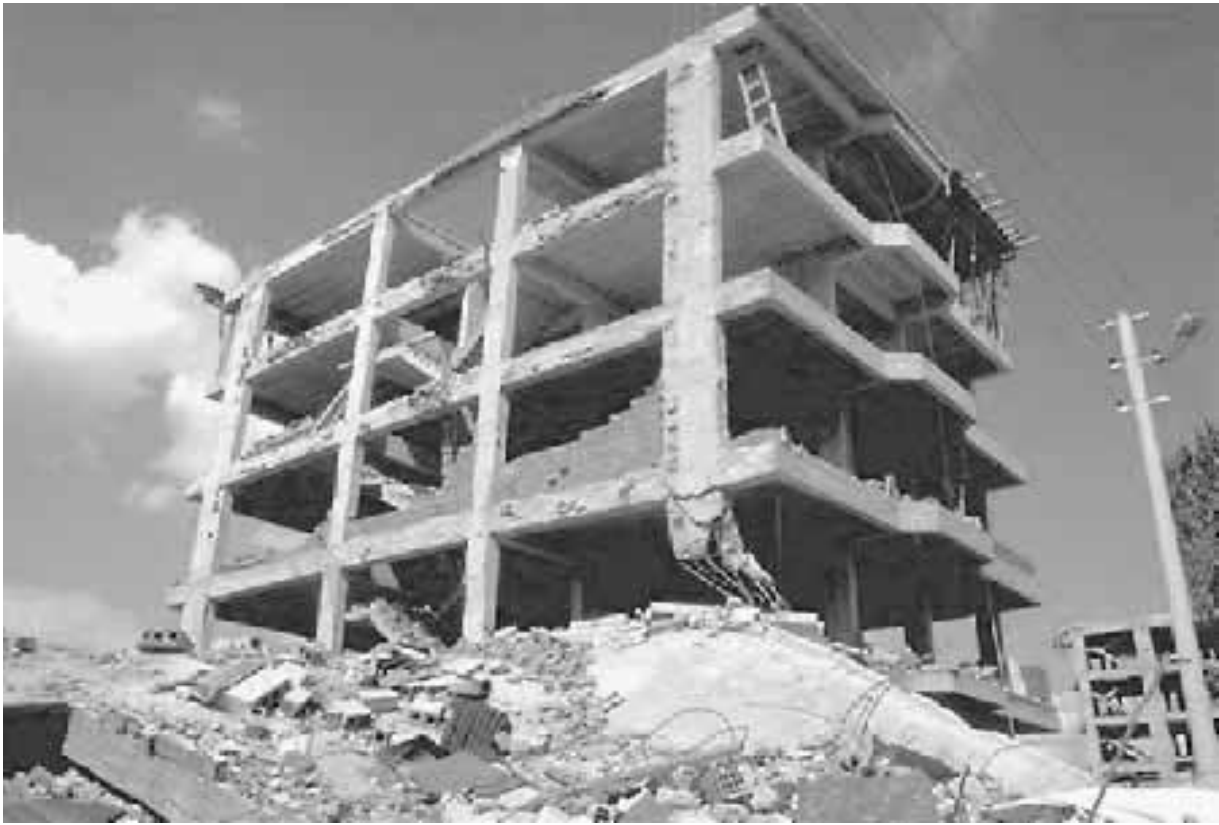
FIGURE 4.22 The building shown has lost a corner column due to the collapse of an adjacent building during the Izmit earthquake in Turkey on August 17, 1999. Note that the roof of the collapsed building now rests on the third-story corner of the standing building. (Photograph from the Izmit Collection, EERC, University of California, Berkeley.)
