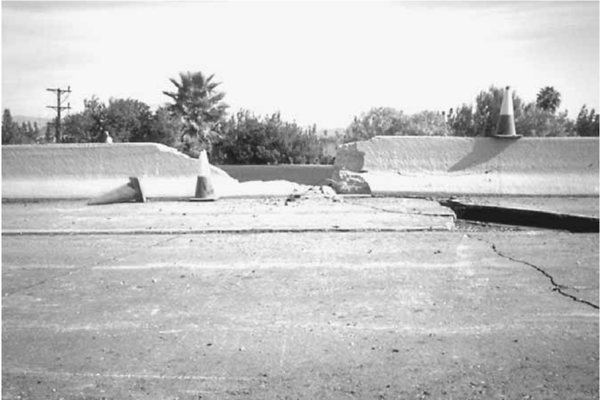
FIGURE 11.4 View to the north along northbound Interstate 405, 250 yards south of Rinaldi Overcrossing. The compressional damage to the roadway and at the median barrier was caused by the Northridge earthquake, in California, on January 17, 1994. (Photograph from the Northridge Collection, EERC, University of California, Berkeley.)
