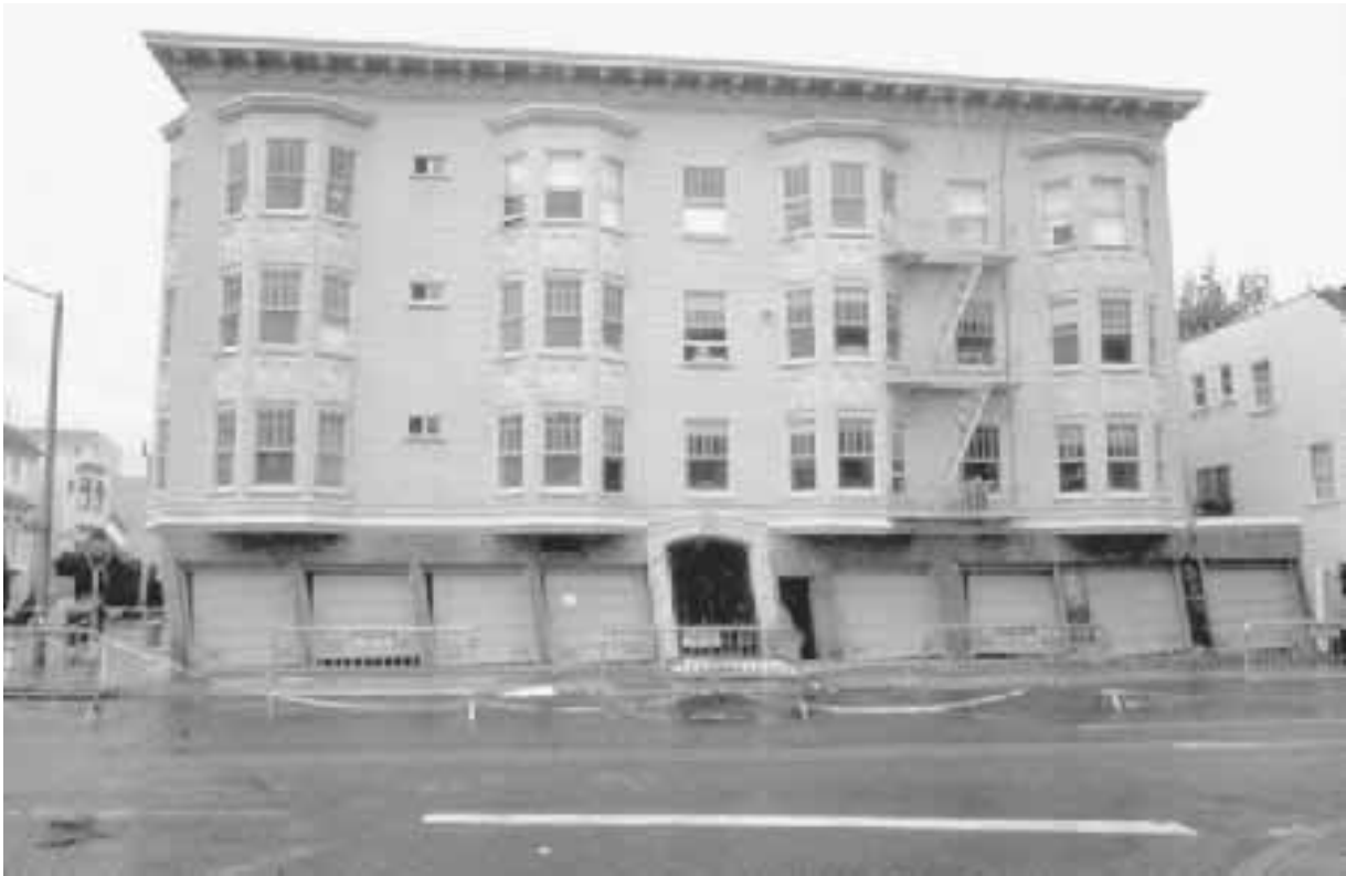
FIGURE 4.8 Damage caused by a soft story due to a parking garage on the first floor. The damage occurred during the Loma Prieta earthquake in California on October 17, 1989. (Photograph from the Loma Prieta Collection, EERC, University of California, Berkeley.)
