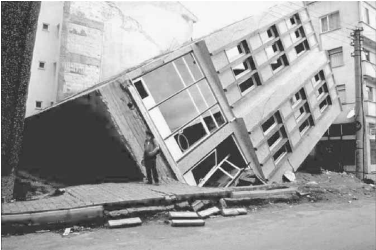
FIGURE 8.4 The building suffered a liquefaction-induced bearing capacity failure during the Izmit earthquake in Turkey on August 17, 1999. (Photograph from the Izmit Collection, EERC, University of California, Berkeley.)
