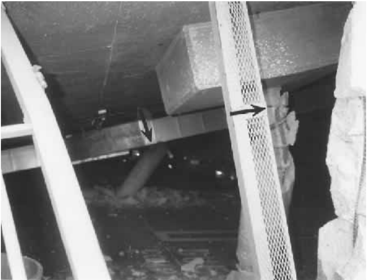
FIGURE 4.7 View inside the collapsed first-floor parking garage (the arrows point to the columns). The building collapse occurred during the Northridge earthquake in California on January 17, 1994.
