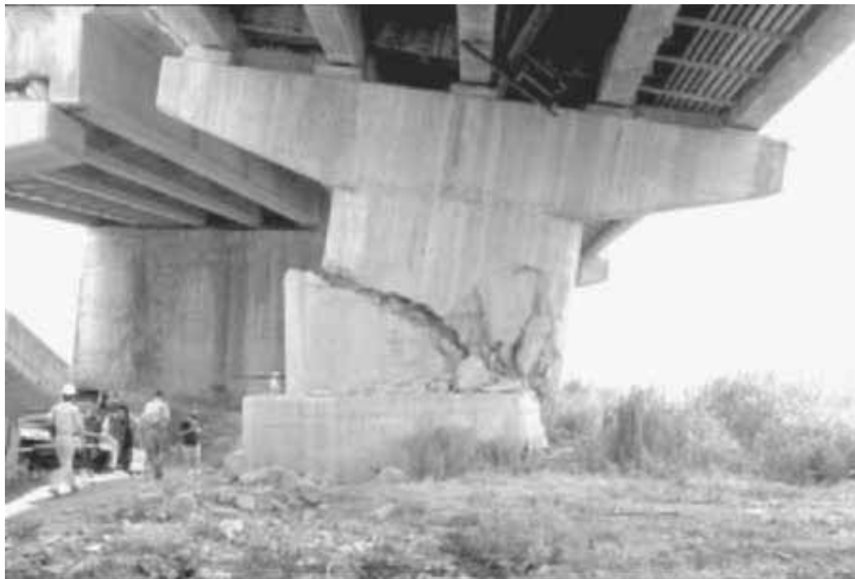
FIGURE 3.7 Close-up view of bridge pier (Wu-His Bridge) damaged by surface fault rupture associated with the Chi-chi (Taiwan) earthquake on September 21, 1999. (Photograph from the Taiwan Collection, EERC, University of California, Berkeley.)
