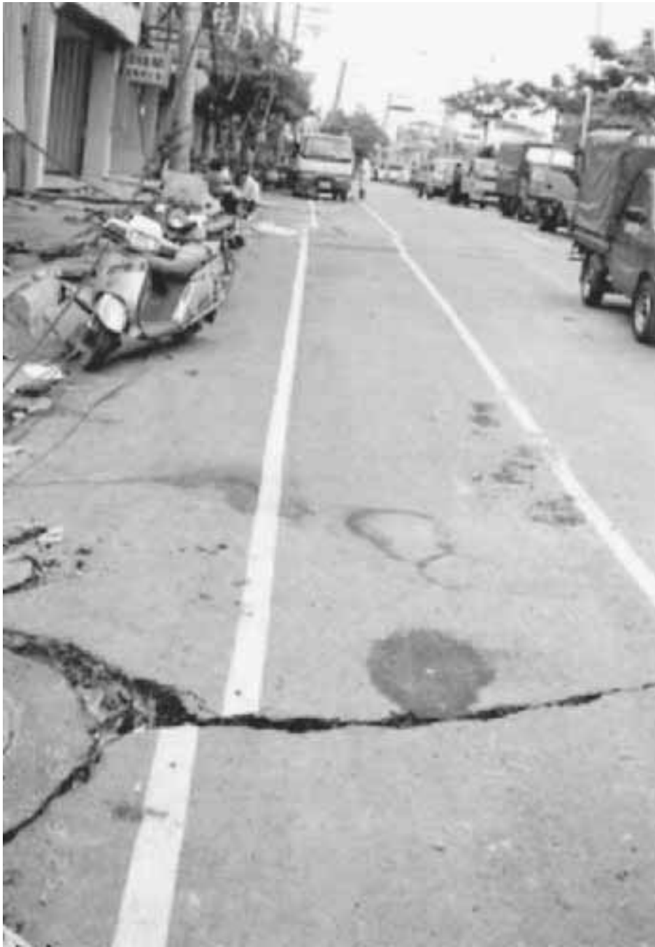
FIGURE 3.13 Surface fault rupture and roadway damage associated with the Chi-chi (Taiwan) earthquake on September 21, 1999. (Photograph from the USGS Earthquake Hazards Program, NEIC, Denver.)
