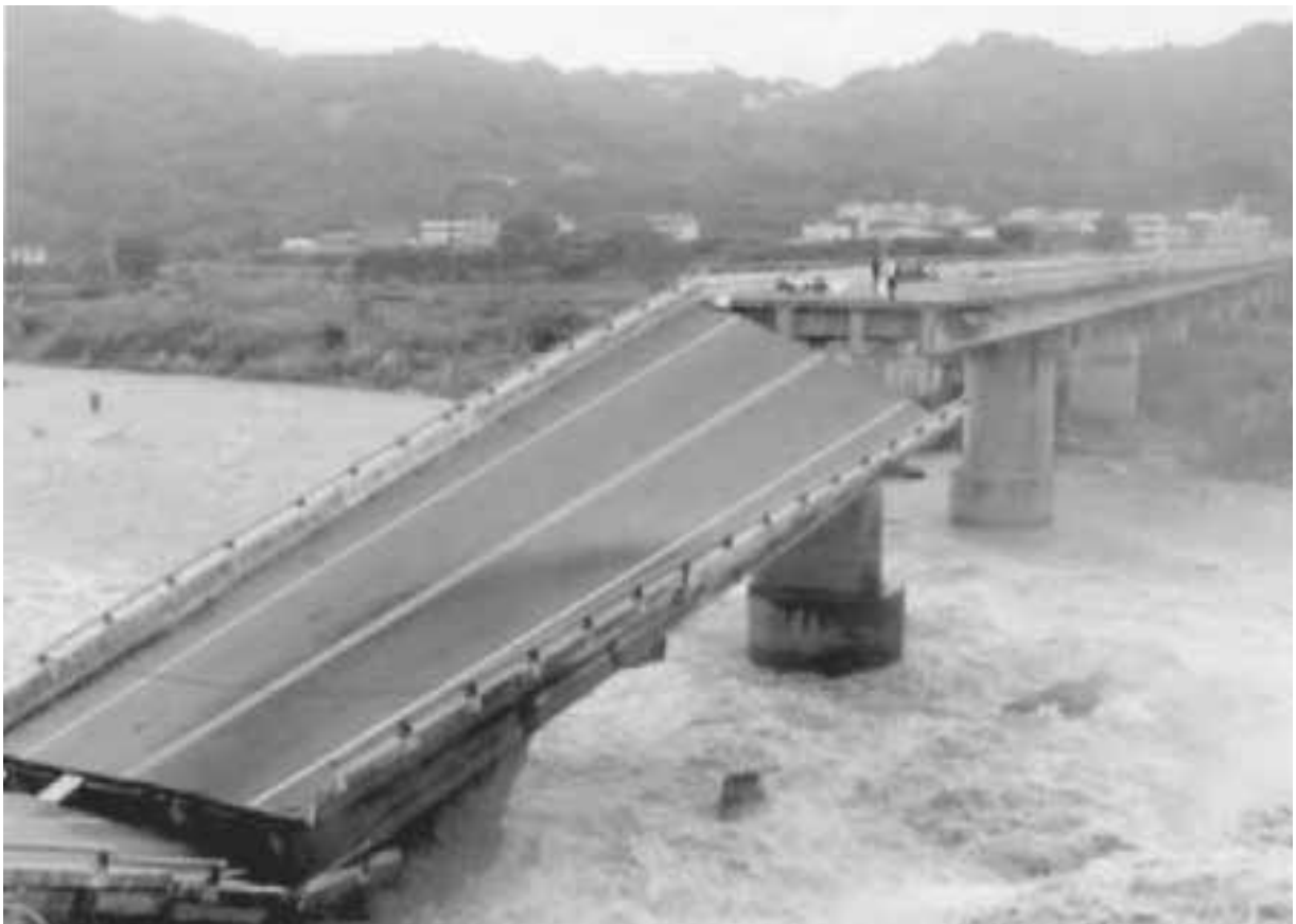
FIGURE 3.9 Collapsed bridge north of Fengyuen caused by surface fault rupture associated with the Chi-chi (Taiwan) earthquake on September 21, 1999. (Photograph from the USGS Earthquake Hazards Program, NEIC, Denver.)
