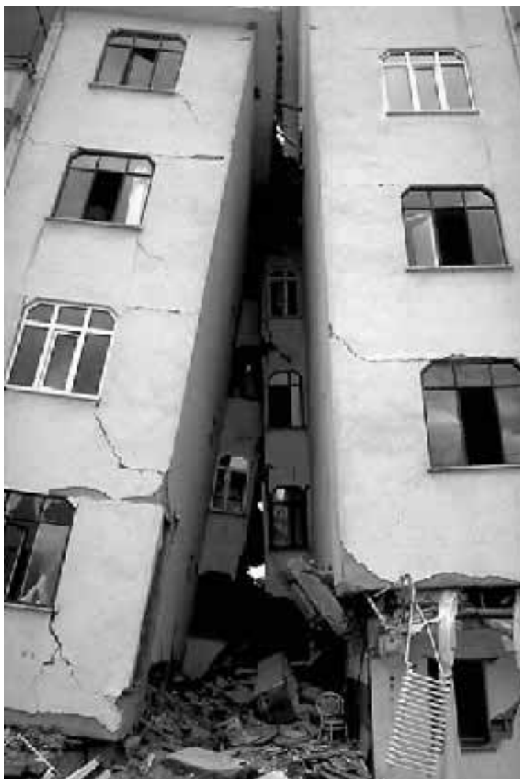
FIGURE 4.21 Another example of pounding damage and eventual collapse caused by the Izmit earthquake in Turkey on August 17, 1999. (Photograph from the Izmit Collection, EERC, University of California, Berkeley.)
