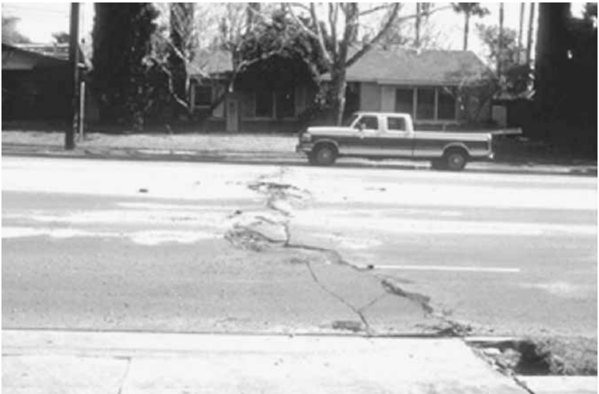
FIGURE 11.5 Localized compression feature and pavement damage caused by the Northridge earthquake, in California, on January 17, 1994. (Photograph from the Northridge Collection, EERC, University of California, Berkeley.)
