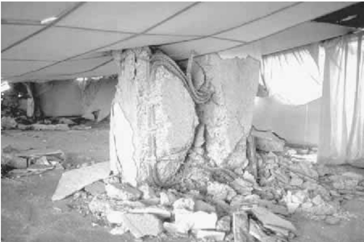
FIGURE 4.4 Close-up view of a collapsed second-story column at the Hotel Terminal. Note that the upper floor has displaced to the right and dropped, and the top and bottom sections of the column are now side by side. The torsional failure occurred during the Gualan earthquake in Guatemala on February 4, 1976. (Photograph from the Godden Collection, EERC, University of California, Berkeley.)
