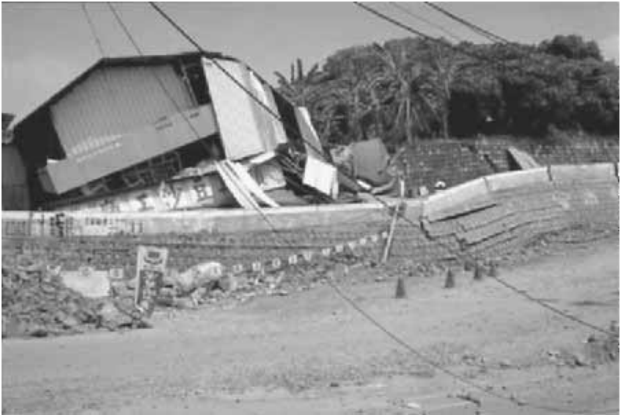
FIGURE 3.8 Retaining wall located north of Chung-Hsing (Jung Shing). At this site, the surface fault rupture associated with the Chi-chi (Taiwan) earthquake on September 21, 1999, has caused both vertical and horizontal displacement of the retaining wall. (Photograph from the Taiwan Collection, EERC, University of California, Berkeley.)
