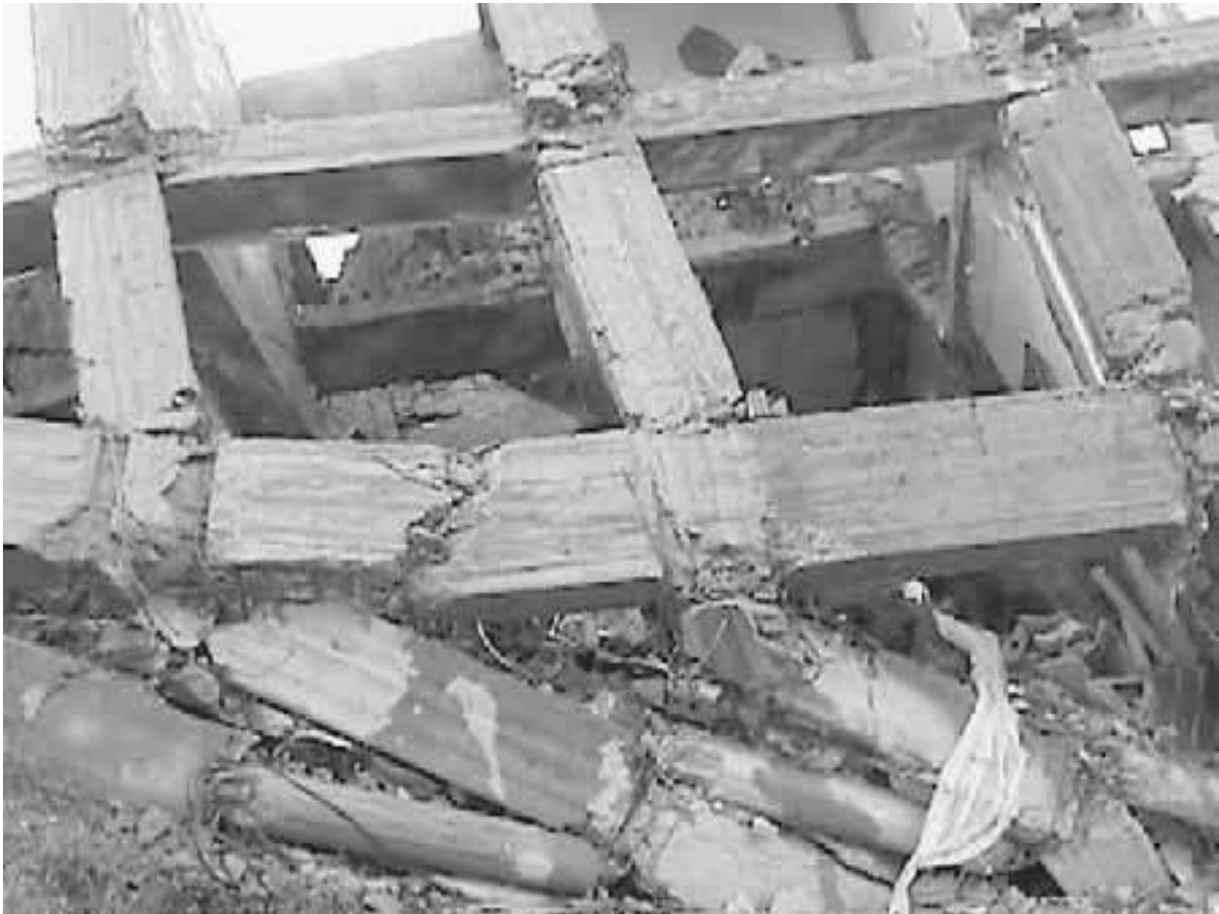
FIGURE 4.10 Building collapse caused by a soft story at the first-floor level. The damage occurred during the Izmit earthquake in Turkey on August 17, 1999. (Photograph by Mehmet Celebi, USGS.)
